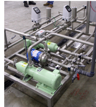
In-line Blending System w/ Magnetic Flow Meters
