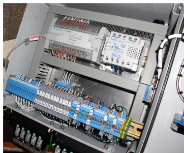
PROCESS LOGIC CONTROLLER
